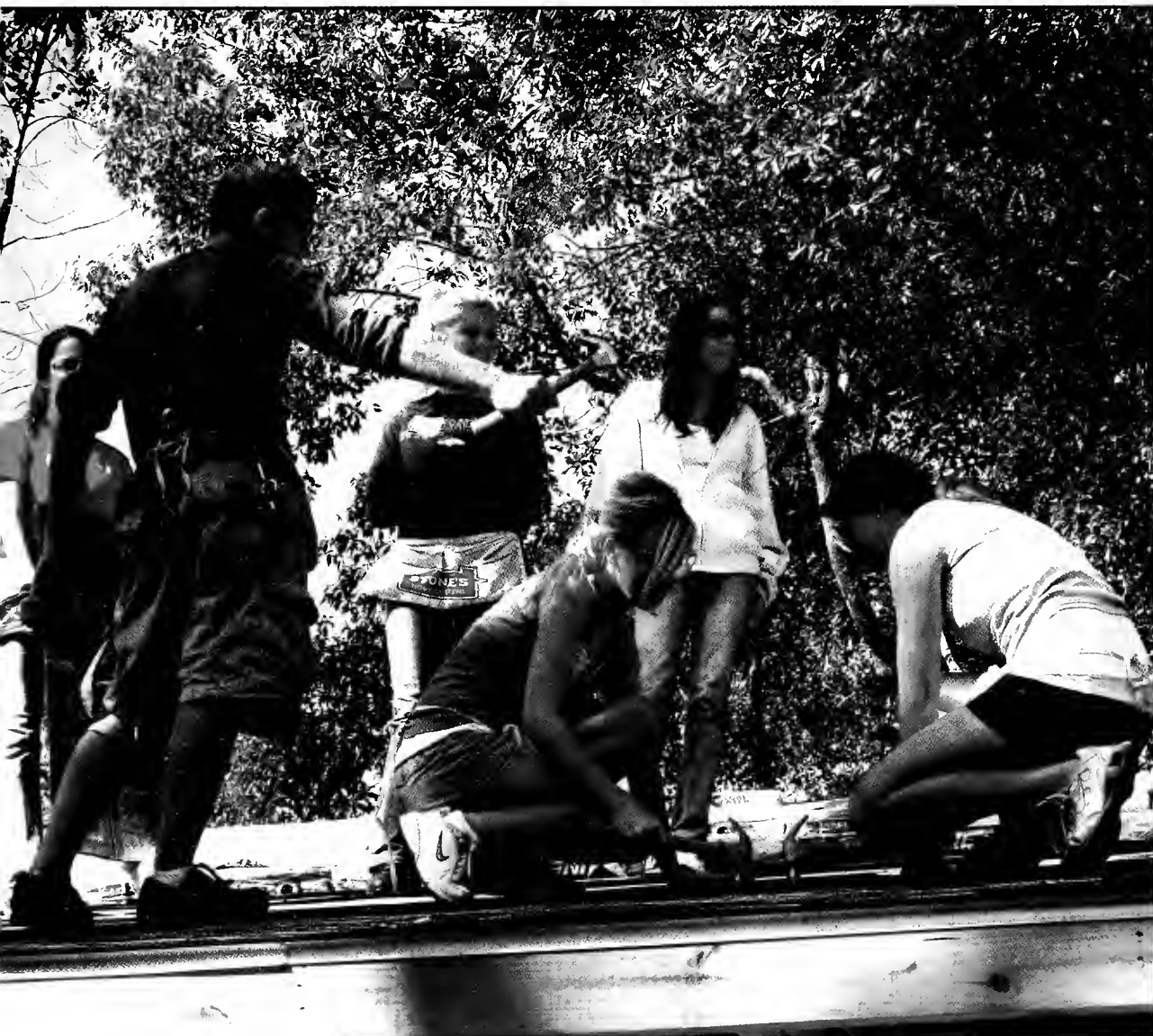
Interior Design students participating in Habitat for Humanity build from IND 3470 Construction Systems, Fall 2007.
